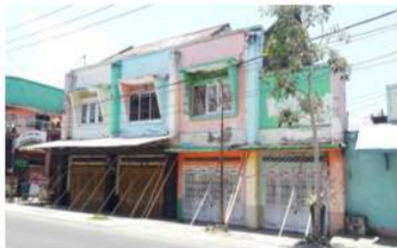
Figure 4. Buildings Damaged by Earthquakes
