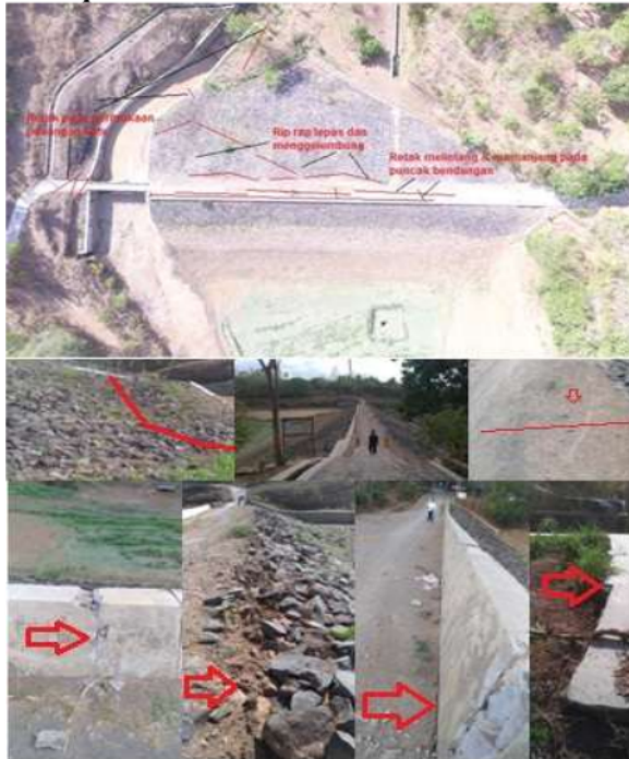
Figure 5 the Gegurik dam after the earthquake
