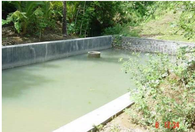
Figure 2. An embung desa with masonry structure as its embankment (Courtesy of BISDA NTB)
