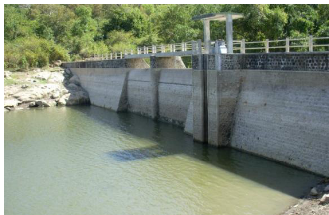
Figure 3. An embung pemerintah equipped with adequate intake and spillway (Courtesy of BWS NT I)
