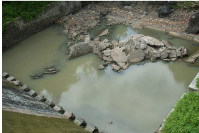
Figure 14. Disintegration of concrete at stilling basin (Courtesy of BWS NT I)
