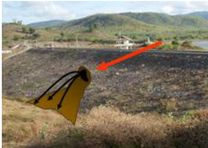
Figure 7. Seepage with mud flow accelerates mass failure (Courtesy of BWS NT I)
