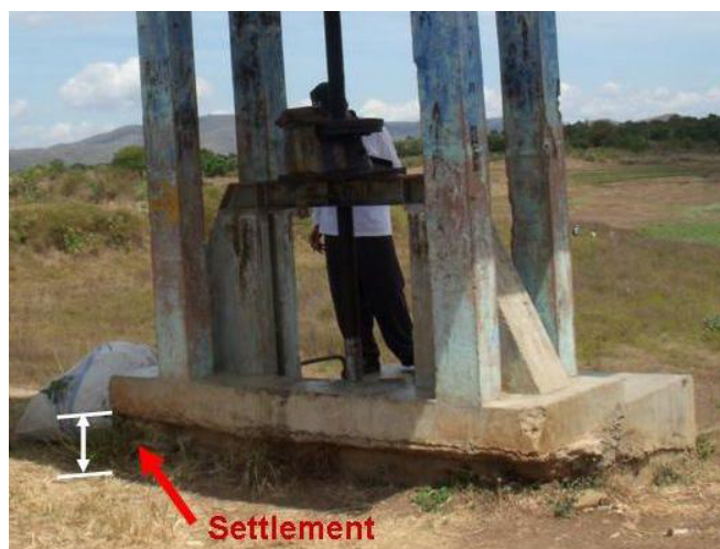
Figure 6. A noticeable settlement of embankment exists around the intake gate (Courtesy of BWS NT I)
