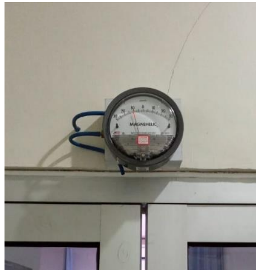
Figure 4. Implanted pressure gauge (magnehelic®)
