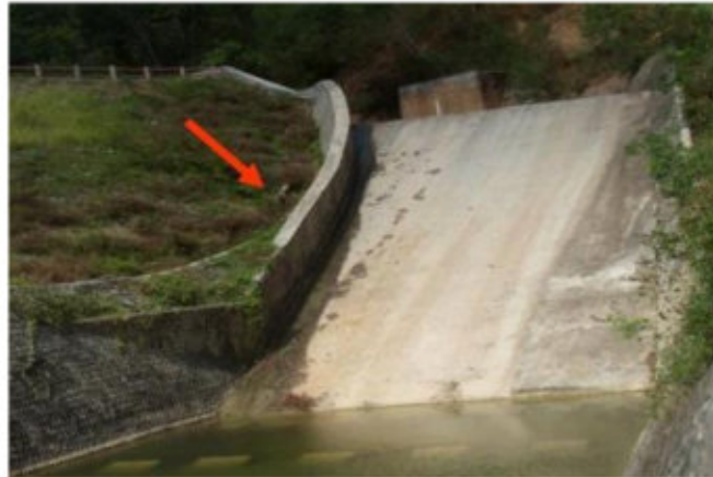
Figure 10. Leakage between embankment and spillway (Courtesy of BWS NT I)
