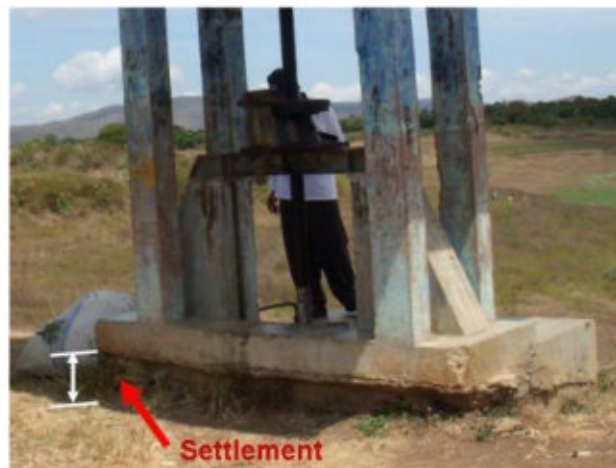
Figure 6. A noticeable settlement of embankment exists around the intake gate (Courtesy of BWS NT I)
