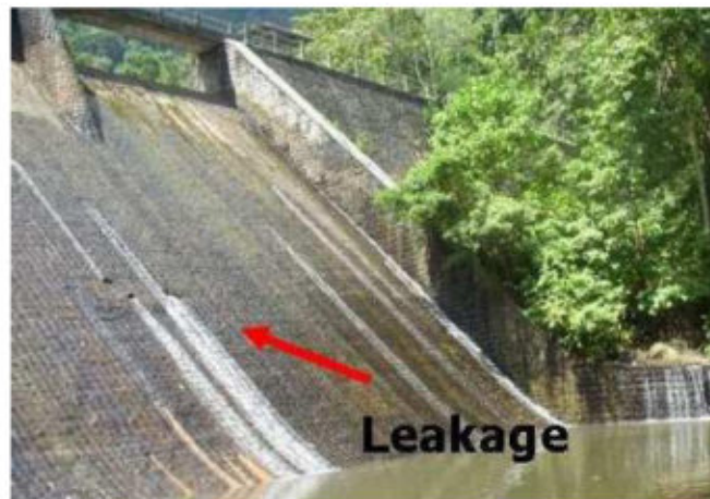
Figure 8. Leakage underneath spillway crest (Courtesy of BWS NT I)
