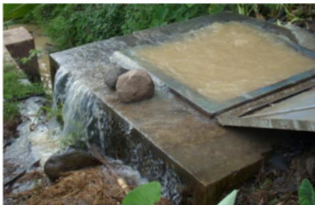
Figure 13. Improper installation of outlet valve (Courtesy of BWS NT I)
