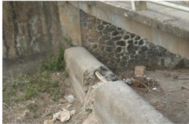
Figure 12. Damages to the spillway crest (Courtesy of BWS NT I)
