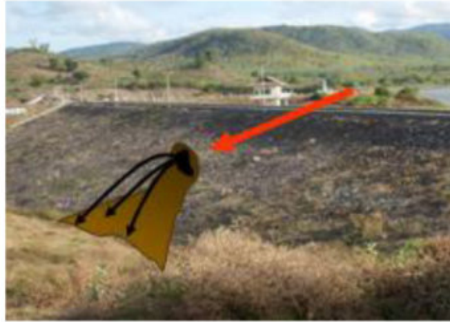
Figure 7. Seepage with mud flow accelerates mass failure (Courtesy of BWS NT I)
