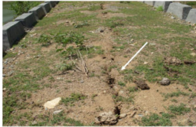
Figure 4. Cracks on top of the embankment (Courtesy of BWS NT I)
