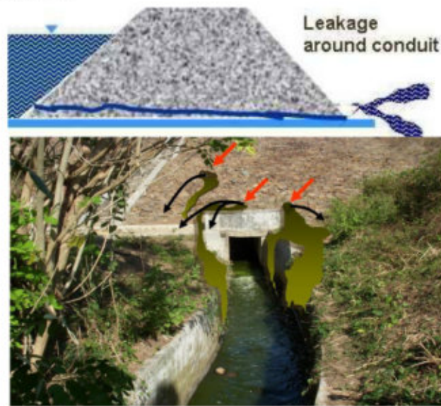
Figure 9. Seepage and leakage around the outlet structure (Courtesy of BWS NT I)
