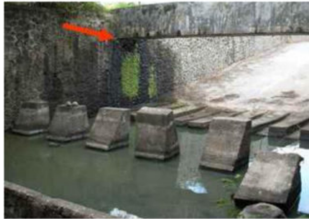
Figure 11. Leakage at the vertical wing wall of stilling basin (Courtesy of BWS NT I)
